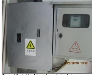
Photo of the inside of the main production hall Electric cabinet.JPG
