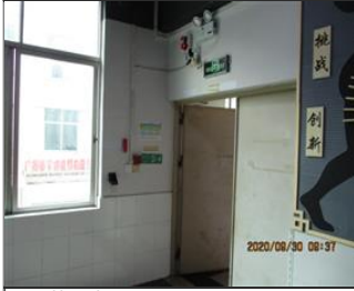
Photo of fire safety equipment Emergency exit.JPG
