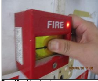
Photo of fire safety equipment Fire alarm test 2.JPG
