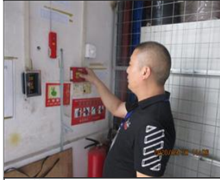
Photo of fire safety equipment Fire alarm test 1.JPG
