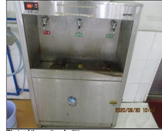
Photo of the sanitary facilities Potable water.JPG
