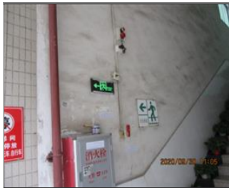
Photo of fire safety equipment Fire equipment.JPG
